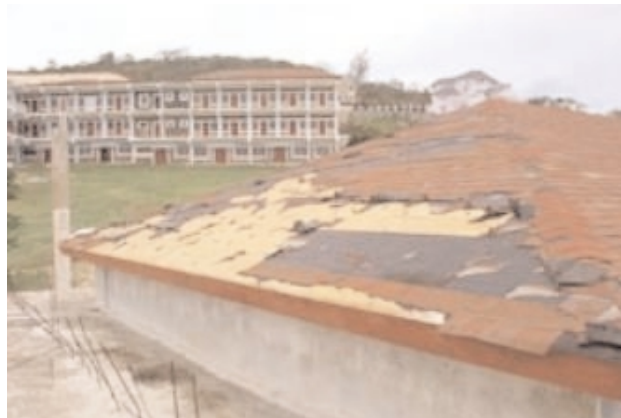
Hurricane Ivan damage to one building at Teamwork Associates.
